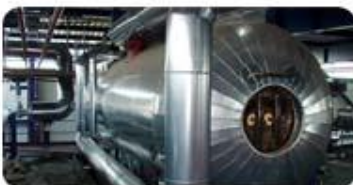
Power Station Insulation
