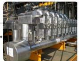
Fuel oil Insulation cover
