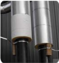
Pipe Insulation Jacketing
