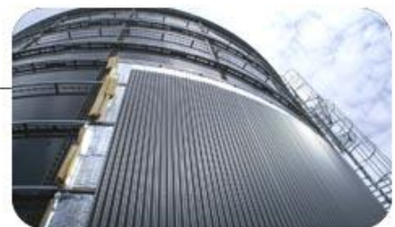
Chemical storage tanks
