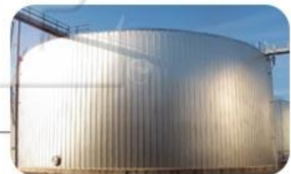
Fuel oil Insulation cover
